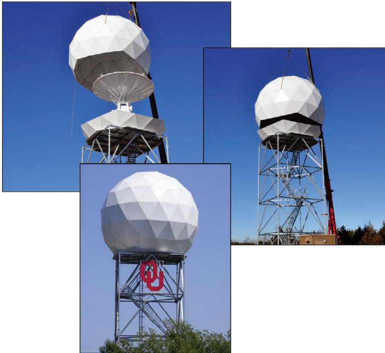
FIG. 6. Photograph of OU-PRIME during the construction phase and after completion in Apr 2009. With a 0.45^\circ intrinsic beamwidth, the radar is one of the highest-resolution polarimetric weather radars in the world.
